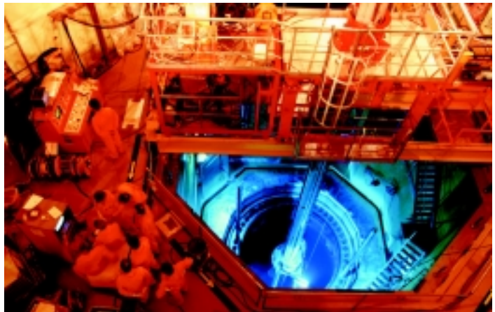
Pressure vessel inspection in a nuclear power station
